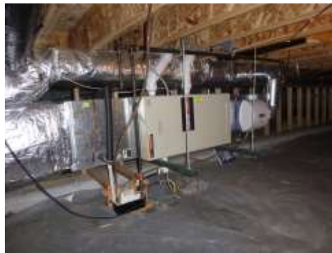
Furnace located in crawl space
