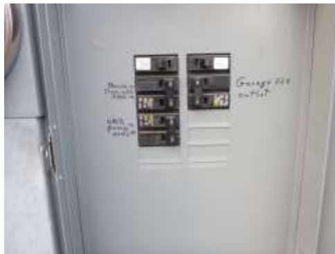
Main breakers in panel
