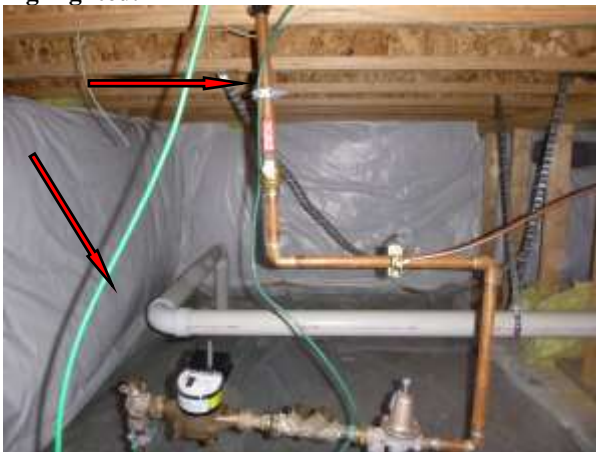
Water main in crawl space with shut off valave highlighted.
