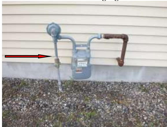
Gas main and shut off valve highlighted.
