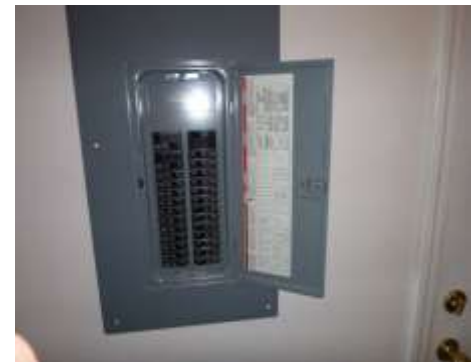
Service panel by garage door
