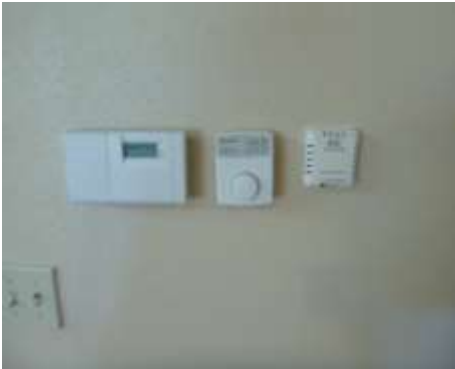
Programmable thermostat on hall wall
